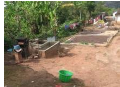
Destroyed coffee processing facility (CPF) and sun drying patio before the project
